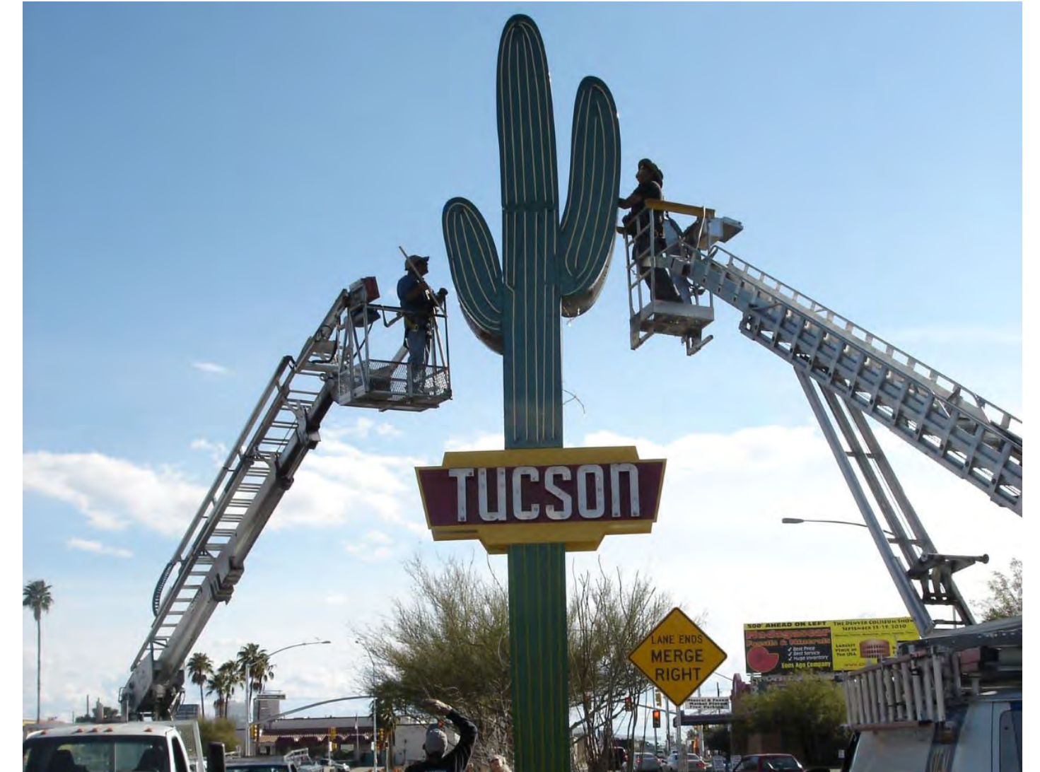
▲ Installation of now iconic 30-ft. Gateway Saguaro public art on Oracle Road in 2009
