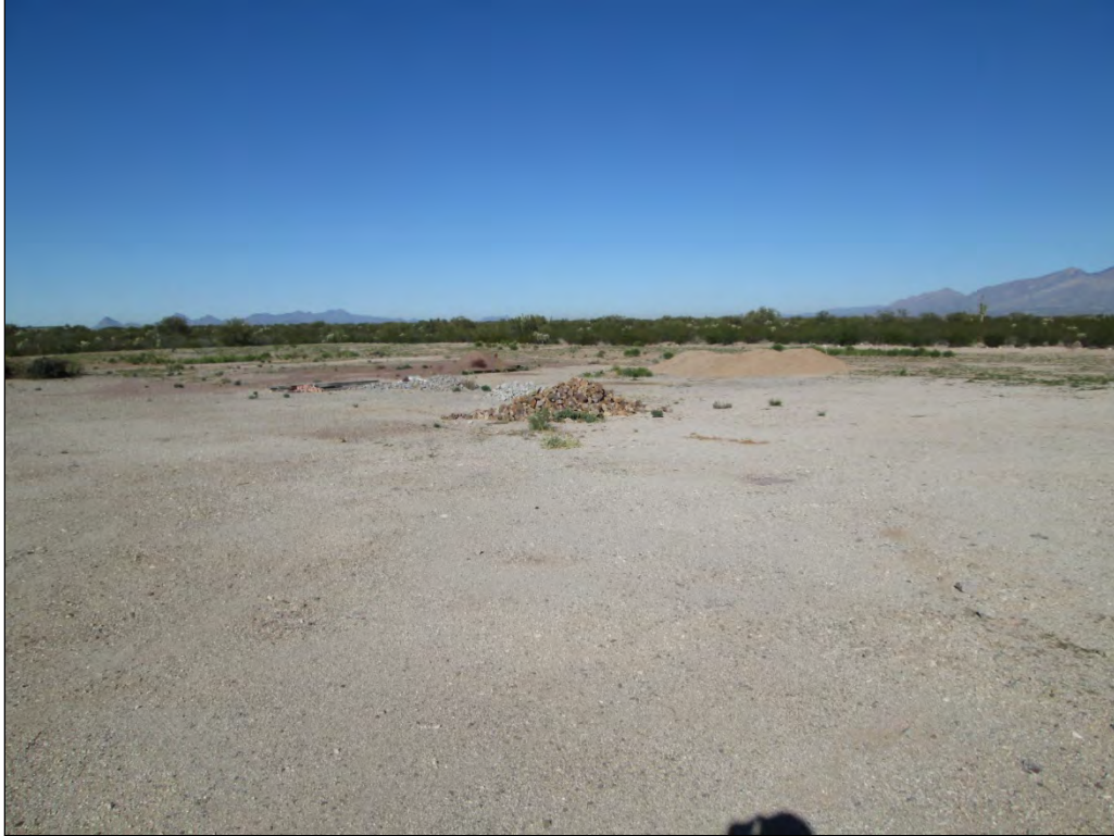
Photo A.1. Project area from the southeast corner showing vegetation clearing and piled materials, looking northwest.
