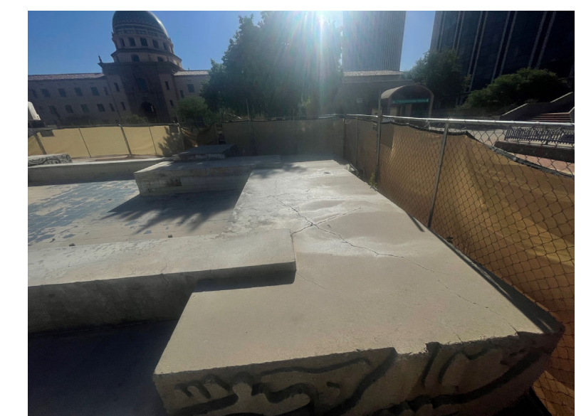
SOUTH-EAST CORNER CONDITION
