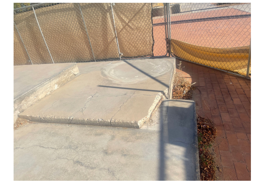
NORTH-WEST CORNER CONDITION
