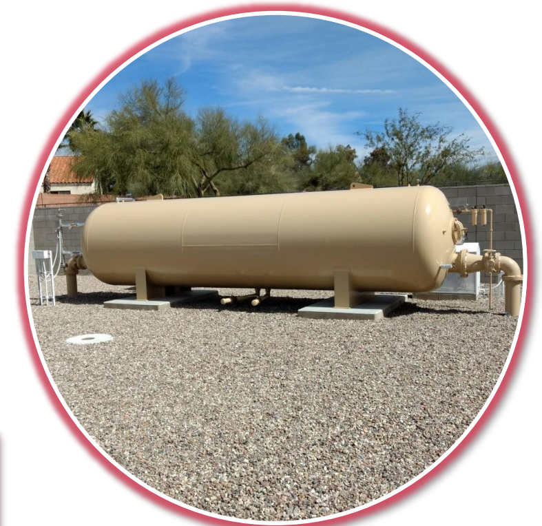
5,000 GALLON HYDRO TANK WITH AIR COMPRESSOR
