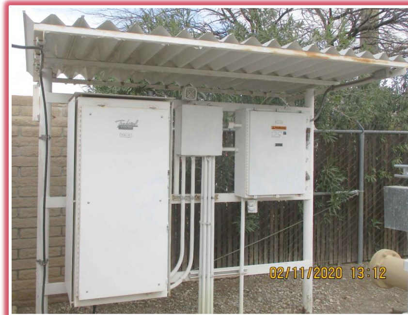
SHADE STRUCTURE WITH ELECTRICAL RACK
