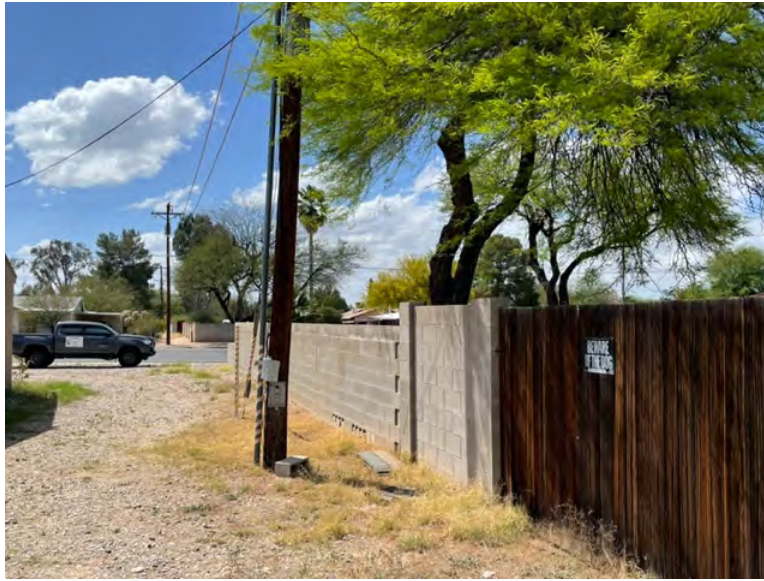
EXHIBIT #22 (Utility Power Pole at the north-east area of the property)
