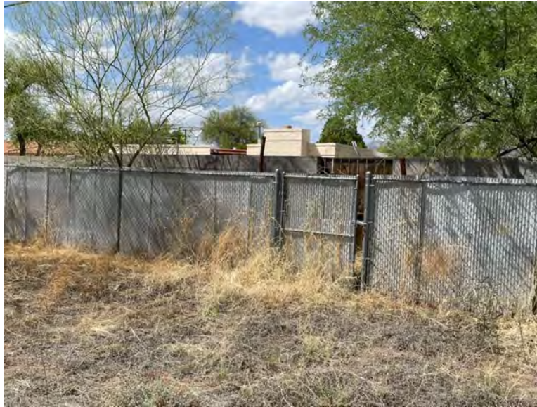
EXHIBIT #15 (Existing North-Fence of the property with chain link fence to be replace by block wall) Wall is outlining the utility easement
