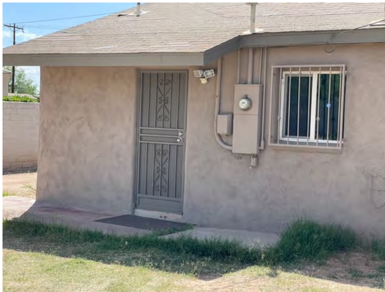
EXHIBIT #25 (Existing Electrical Panel)
