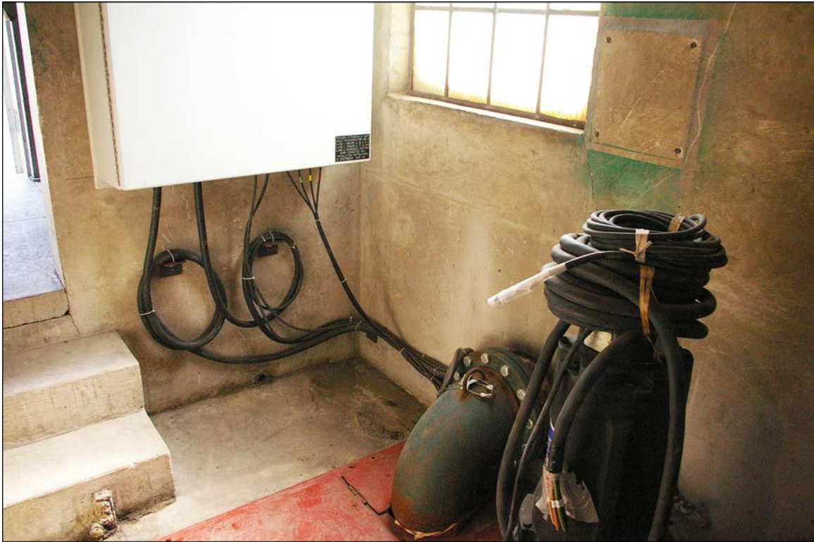
Figure 24. Interior of pump house, Parcel Number 117-05-068F; view to the northeast.
