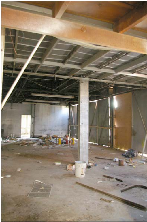
Figure 16. Interior of service building, 503 N. Stone Avenue, showing metal- and wood-frame components of the roofing system; view to the east-southeast.
