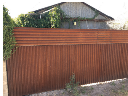
3 Example of weathering corrugated steel
