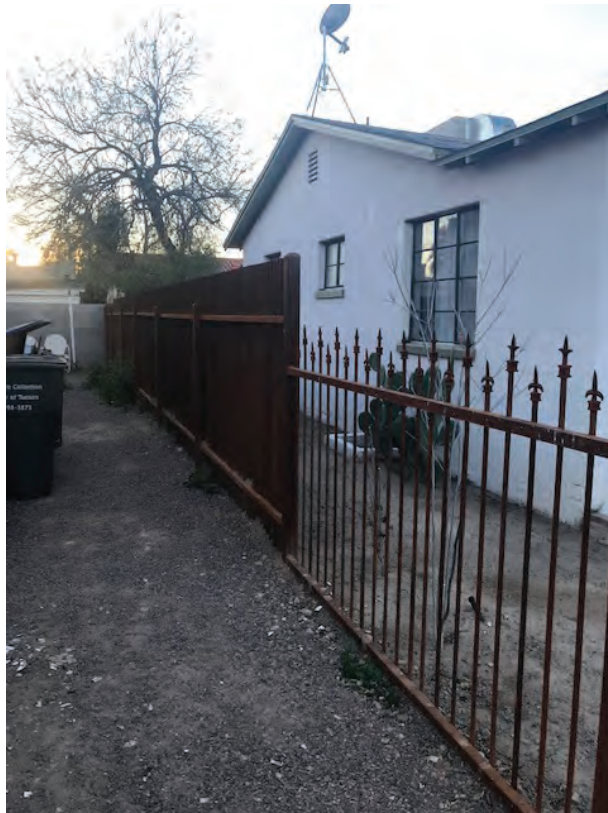
736 SOUTH HERBERT - NEW CONSTRUCTION RUSTED CORRUGATED FENCE
