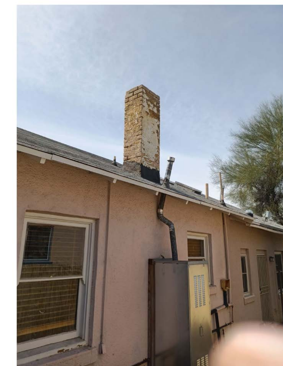
#4 Remove Existing stucco-brick chimney to ground, creating interior space for WH. Replace with stucco-framing chimney to match original.
