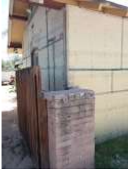
Original pillar on west face north end of guest house / garage (Arizona Ave)
