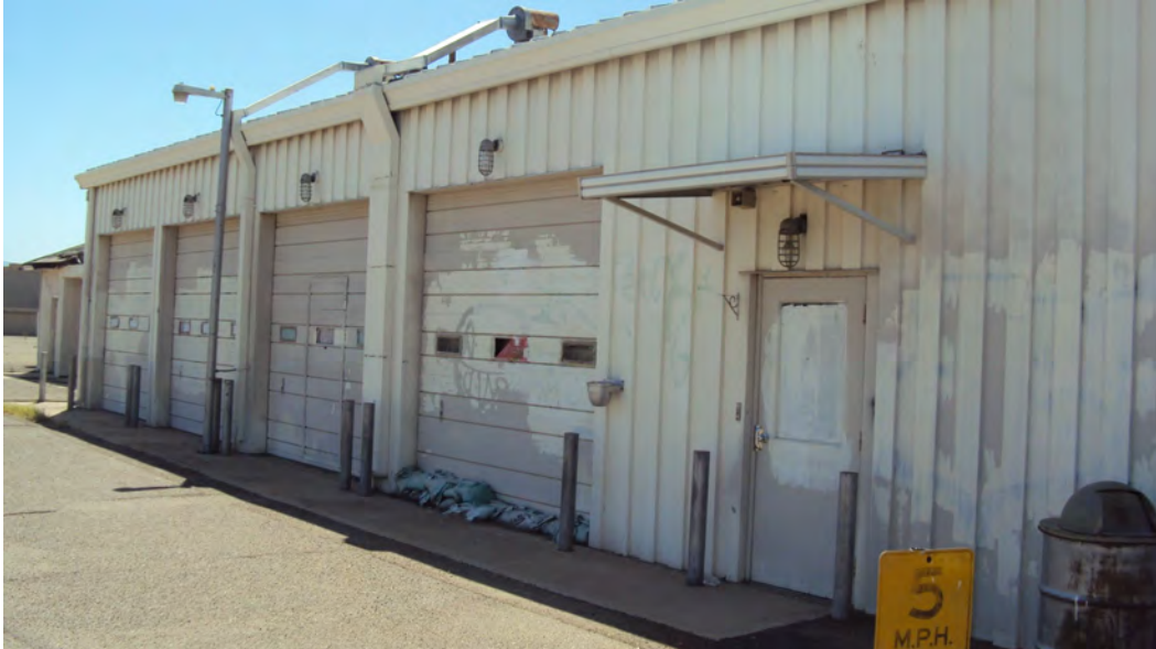
Photo 10: Looking Southwest at the building on the subject parcel from the sidewalk located adjacent (west) to the subject parcel.
