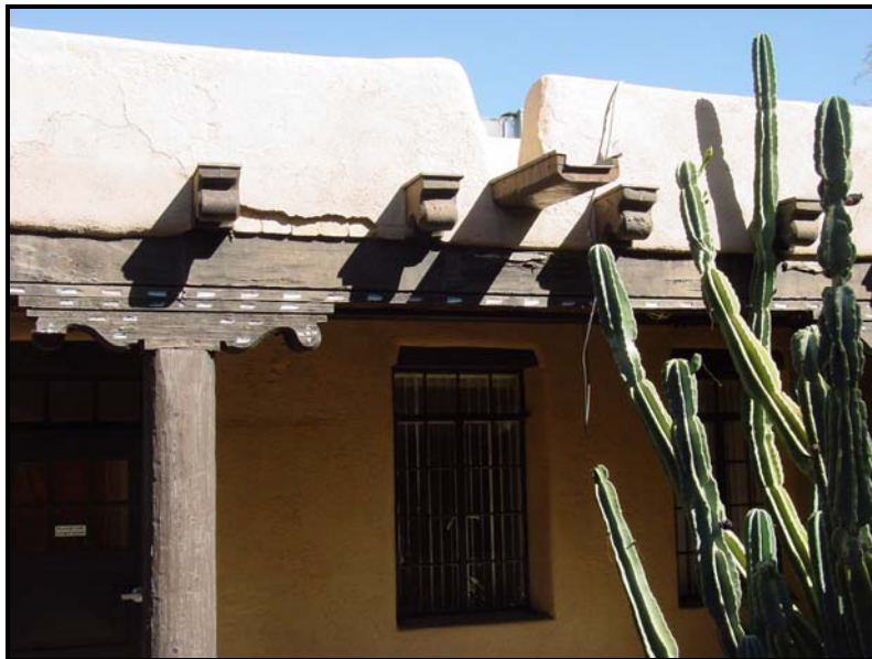
Photograph 12. Detail of parapet and loggia posts at the Patio Building, looking northeast (2009).
