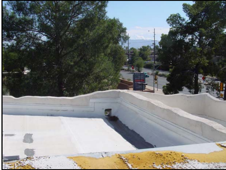
Photograph 20. Southeast corner of the Arizona Building, roof and parapet detail, looking southeast (2009).
