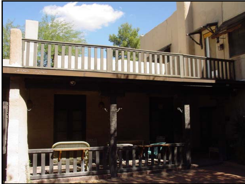
Photograph 34. Detail of porch on south elevation of the Erickson Residence, looking northeast (2009).
