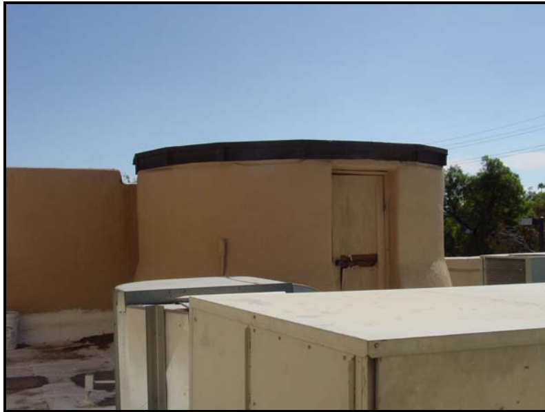
Photograph 10. Base of former radiometer at the southeast corner of the Patio Building, looking southeast (2009).
