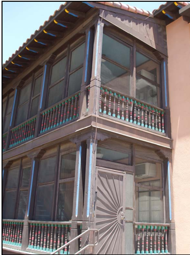
Photograph 28. Sleeping porch detail of nurse's north residence, Veteran's Administration Hospital No. 51, viewing facing north-northeast (2010).
