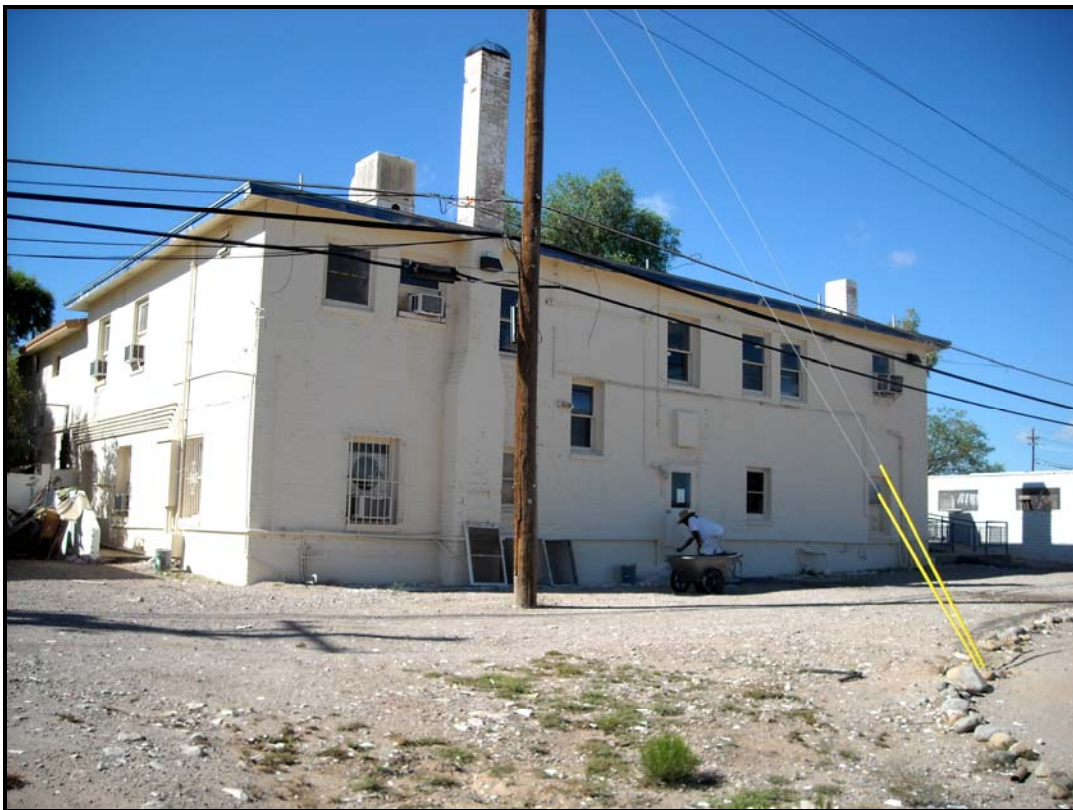
Photograph 57. Former patient ward and incinerator at Arizona State Elk's Association Hospital (near northeast corner of building), view facing southwest (2010).
