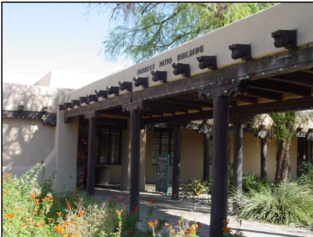
Photograph 16. Detail of west elevation loggia, Patio Building (Desert Sanatorium), view facing north (2010).
