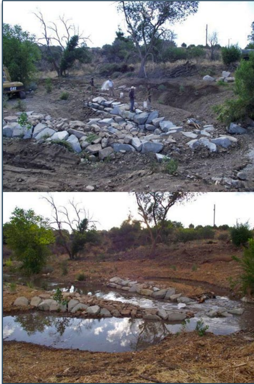
Figure 3.31. During- and post-construction of a large Zuni bowl. Source: Stream Dynamics, Inc.
