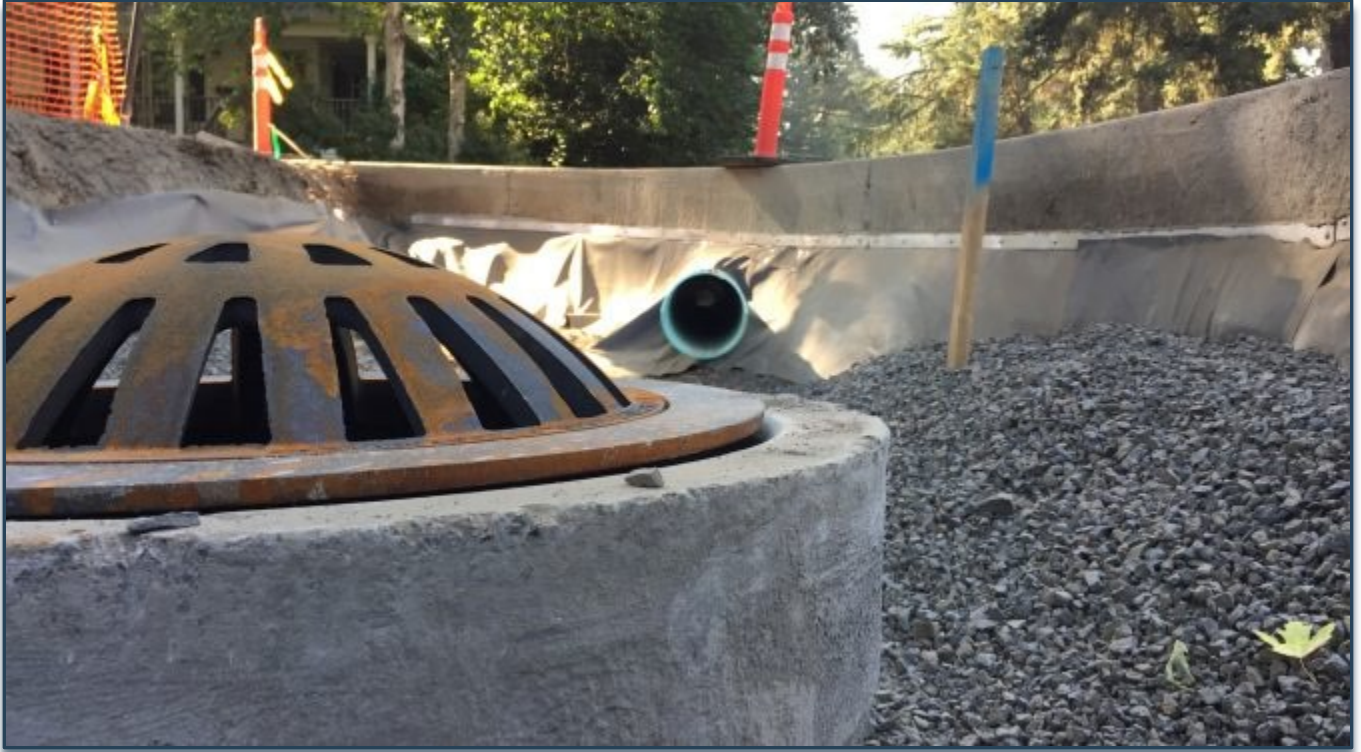
Figure 3.6. Dome overflow with riser. Source: City of Lake Oswego, D Avenue Improvement Project.
