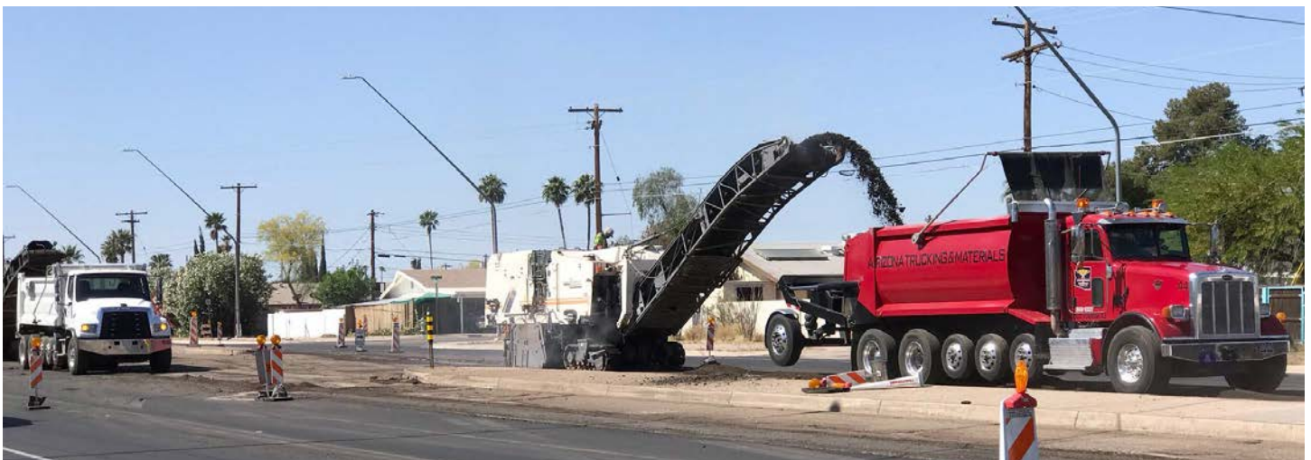
An asphalt milling machine removes the top layer of asphalt on Wilmot Road north of Golf Links.
