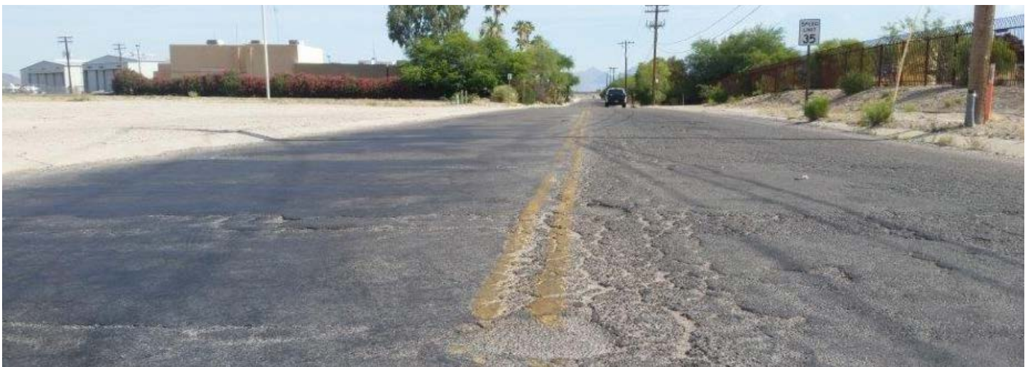
Plumer Avenue before repaving.
