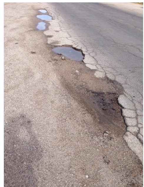
Increased pavement damage without curb.
