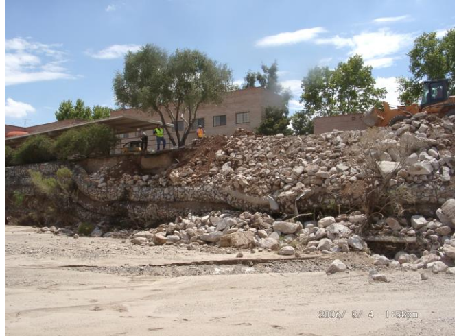
Figure 34: Flooding can easily damage city infrastructure
