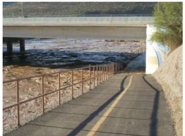
Figure 38: Santa Cruz River Bike Lane Underpass – flooded
