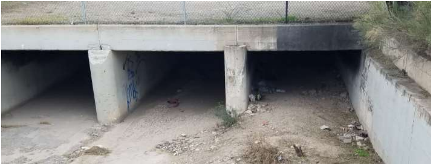
Figure 39: Blackened concrete at location where encampment was removed from box culvert after a fire.
