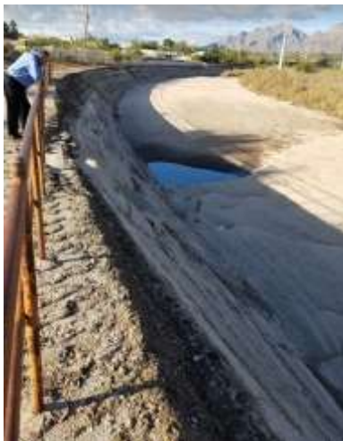
Figure 10: Rillito regional watercourse soil cement embankment with railing and naturally sandy bottom.
