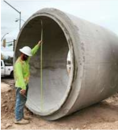
Figure 30: Broadway Boulevard Project includes installation of sixteen 90-inch diameter underground storm drains as part of the Broadway Improvement Project from Euclid Ave to Country Club Road including approximately 192 tons of stormdrain pipe installed in one day.
