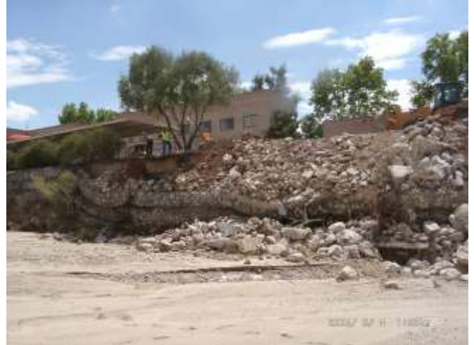
Figure 51: Flooding can easily damage city infrastructure
