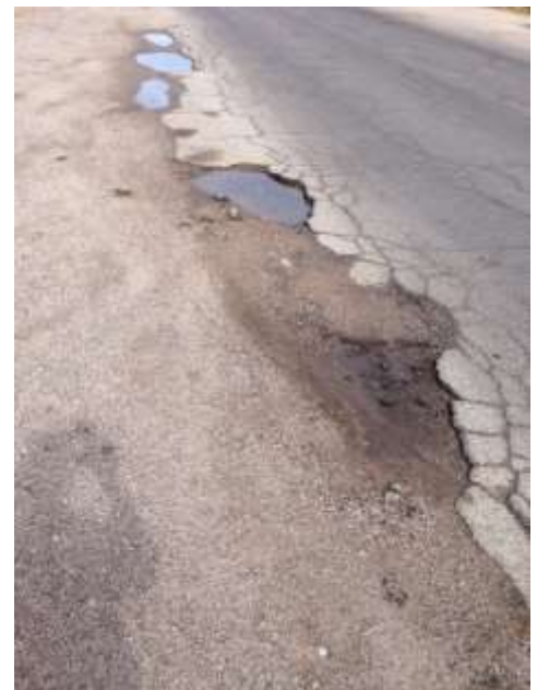
Figure 22: Increased pavement damage without curb.
