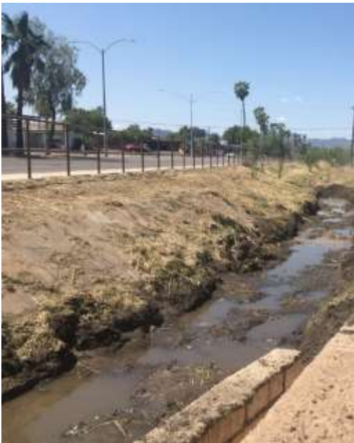
Figure 36: Maintenance is needed to re-establish flowline.
