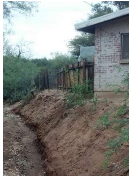
Figure 43: Erosion Hazards can cause structural issues
