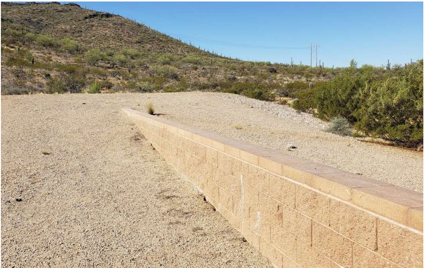
Figure 41: Floodwall Levee on the Silvercroft (ERZ) watercourse at termination point (see page 39)
