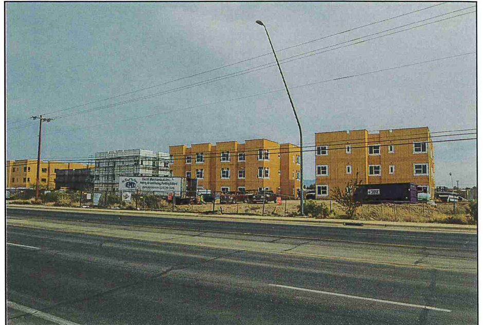
PHOTO 14: Northeast-facing view of the residential apartment complex under construction on adjoining property to the northeast.
