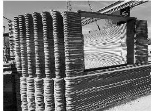
The first home constructed by Habitat for Humanity using 3D printing in Tempe, Arizona
