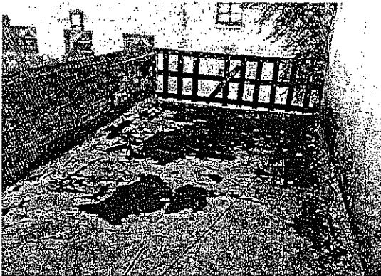
Hole in balcony.
