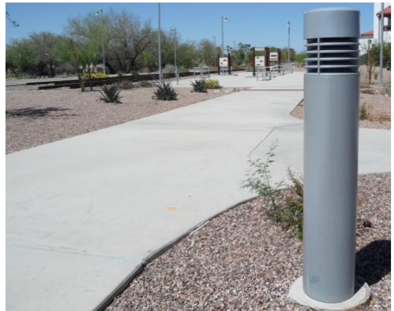
Pedestrian Pathway Lighting
