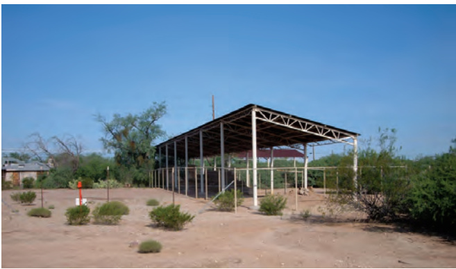
Figure 79: The existing protective roof covering the adobe walls at the Cavalry Corral should be removed.
