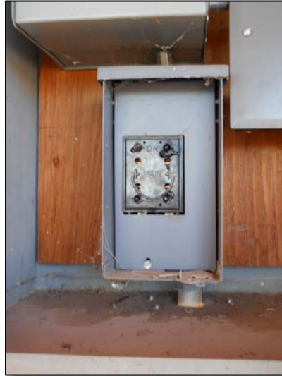
Melted "Pull-Out: Fuse Holder
