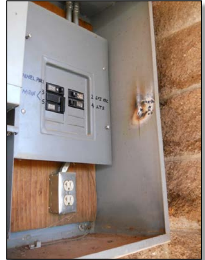
Arc Flash Burn within Cabinet
