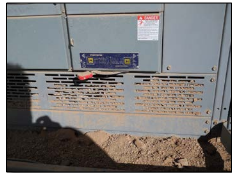
Dirt Accumulation within Cabinet
