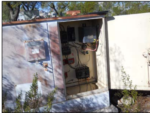
Lower Kennedy Park Service Distribution
