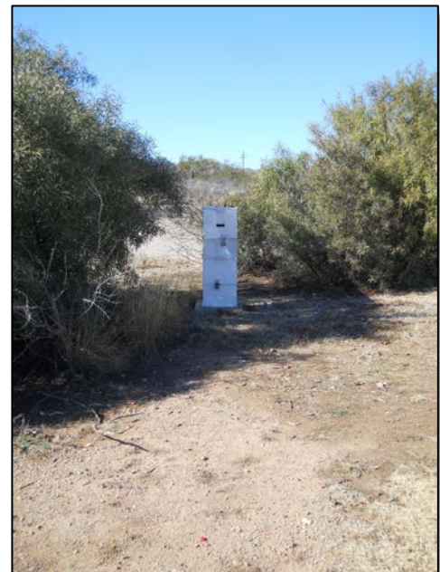
Ramada 33 Service Pedestal
