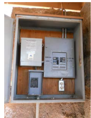
Upper Kennedy Ramada Distribution Cabinet
