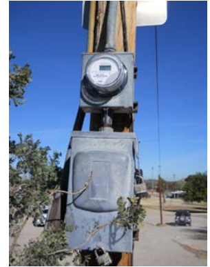
Electrical Compound Service Disconnect
