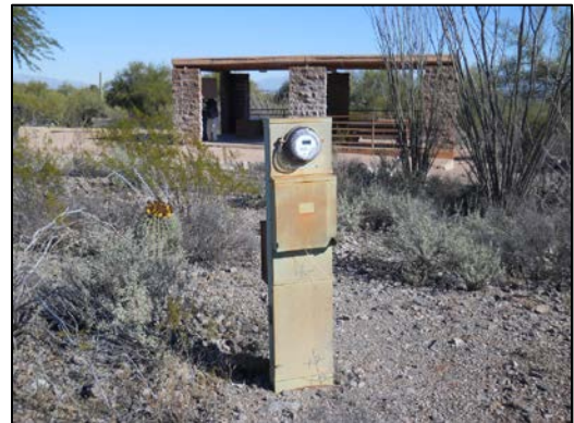
Upper Kennedy Second Service Distribution (Far West Ramadas)
