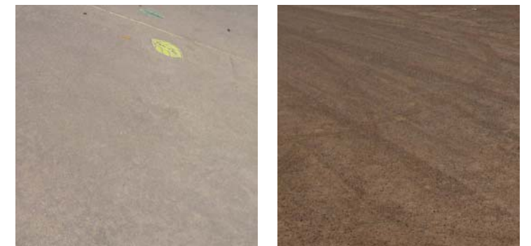
Paving materials clockwise from top left: Exposed Aggregate Finish Integral Color Concrete, Stabilized Aggregate Pavement, Stabilized Decomposed Granite, and Etched Finish Integral Color Concrete with Tile Inserts Photos: WSA
