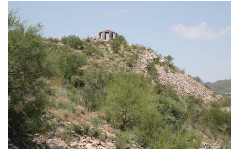
Erosion below existing Ramada Photo: WSA, 2008
