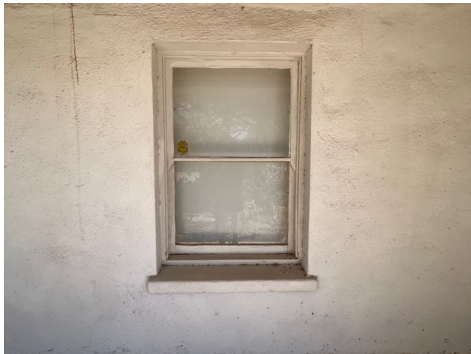
Looking South at the 5215 E Fort Lowell Rd building same window type and detail, note wall texture.
