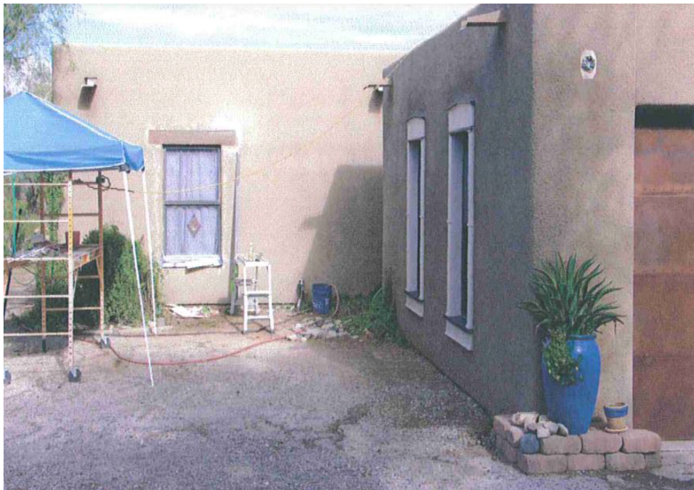
Looking North showing window type and detail along with wall type and texture, and canale type.
