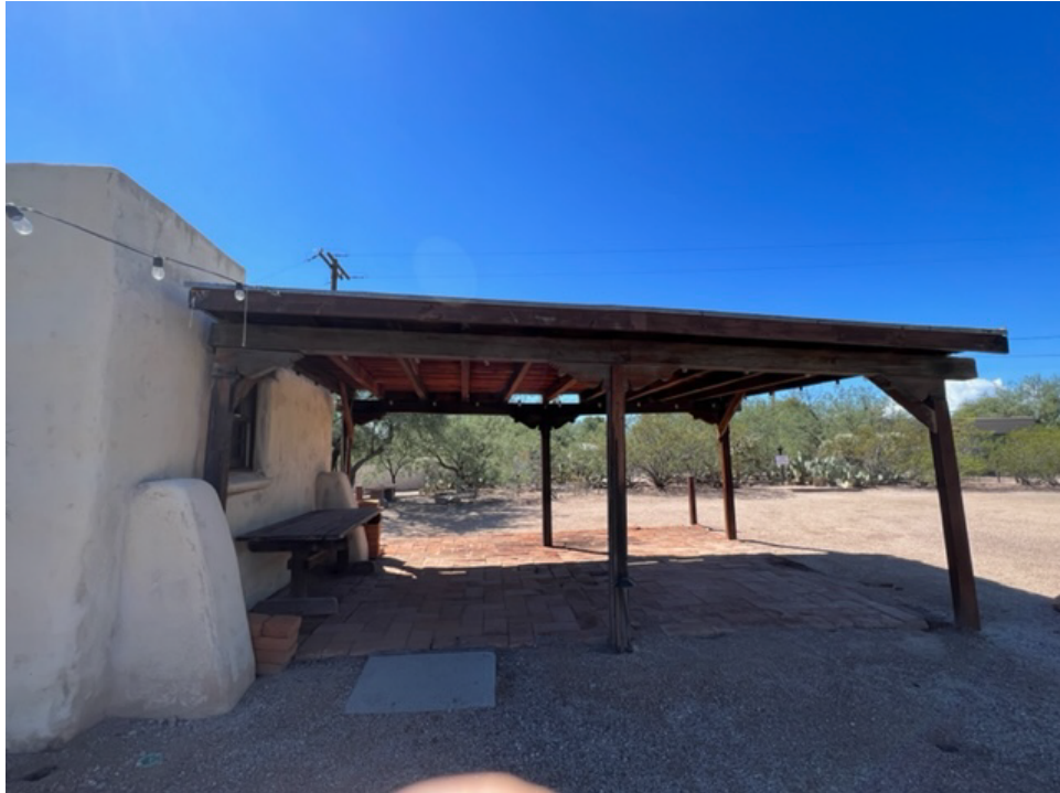
Looking West showing attached structure to the building, detail of wood framed Ramada with pavers.
