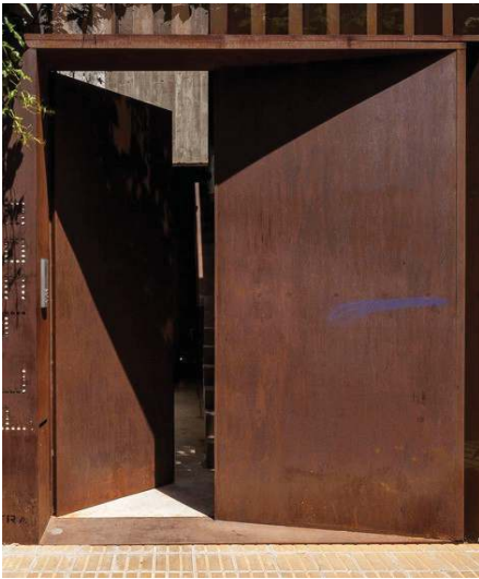
Rusted Metal Double Door Entry Courtyard
