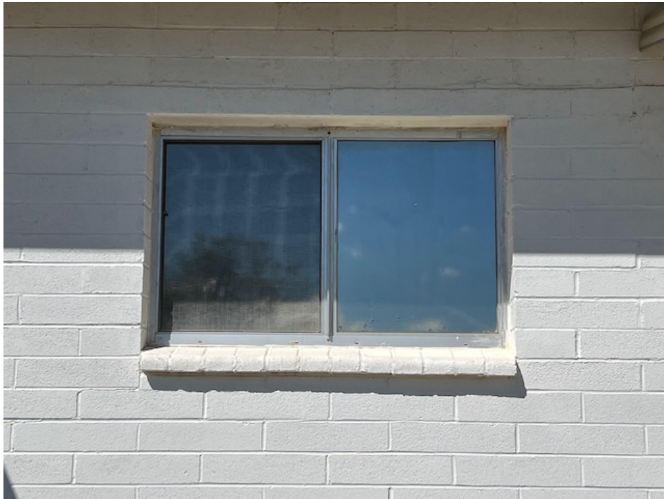
Looking East at the 5215 E Fort Lowell Rd building same window type and detail, note wall texture.
