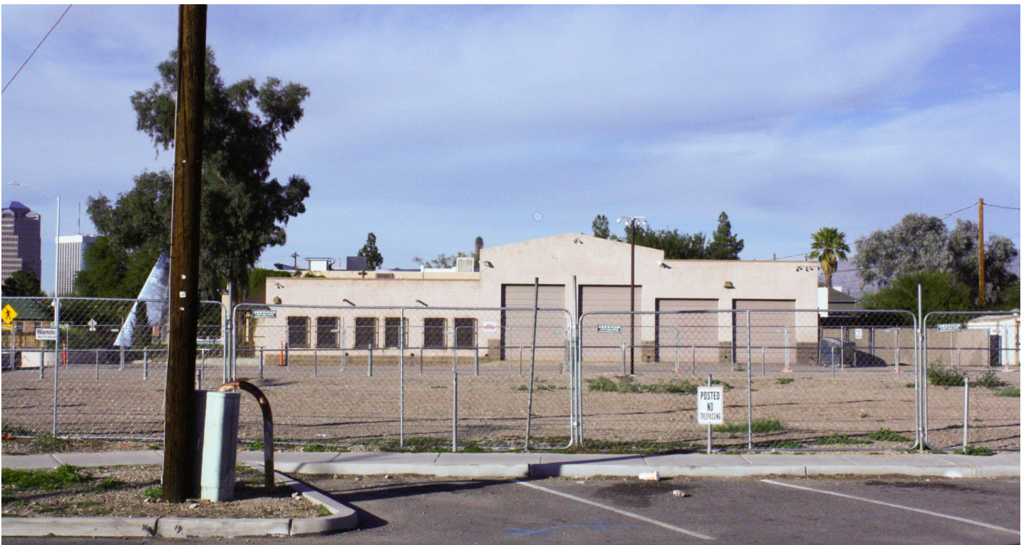
(4) Baffert project site (under construction) and the Wanslee property to the north.
