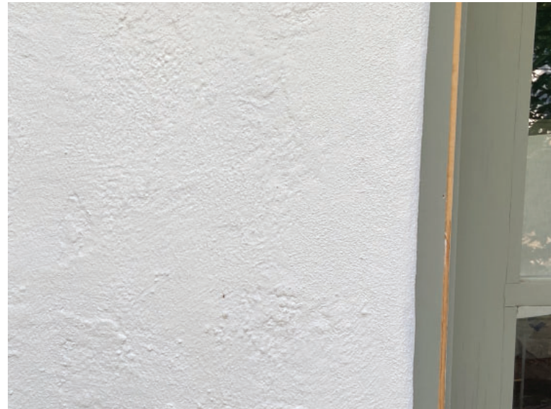
Stucco color and texture of existing main house Window color to right of image
