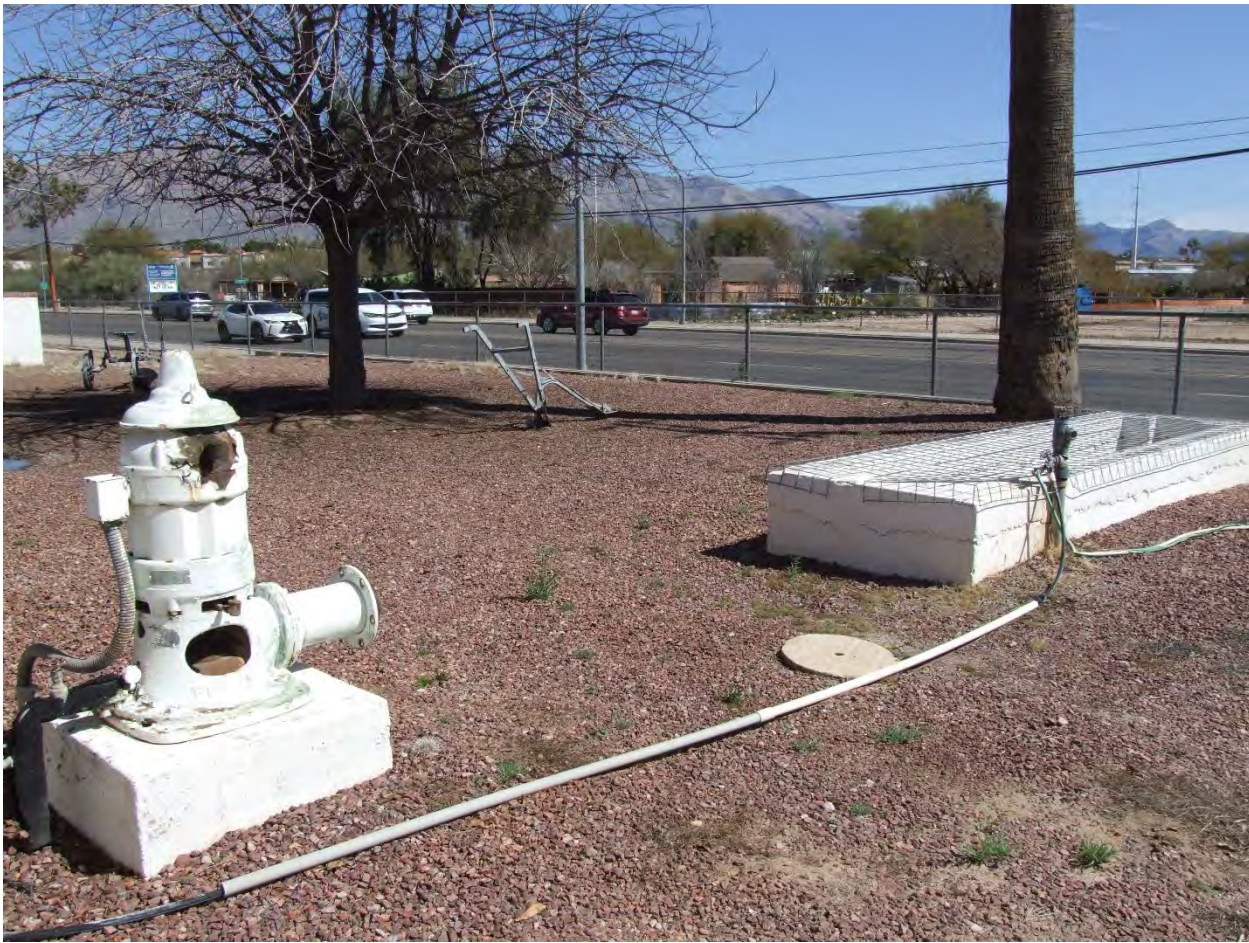
The University of Arizona Agricultural Center, Details of water pump and water holding tank, view facing northeast. WestLand Resources, Inc., March 8, 2023.
