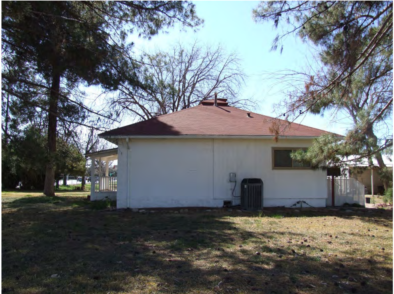
Photograph 4. Overview of north elevation of the Residence; view facing south (UA_Pima County_UA Campus Agricultural Center Historic District_0004).
