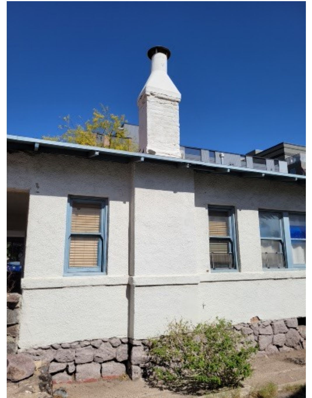
West elevation, noting tufa foundation, 5.5" sill course and brick chimney extending above roofline.
