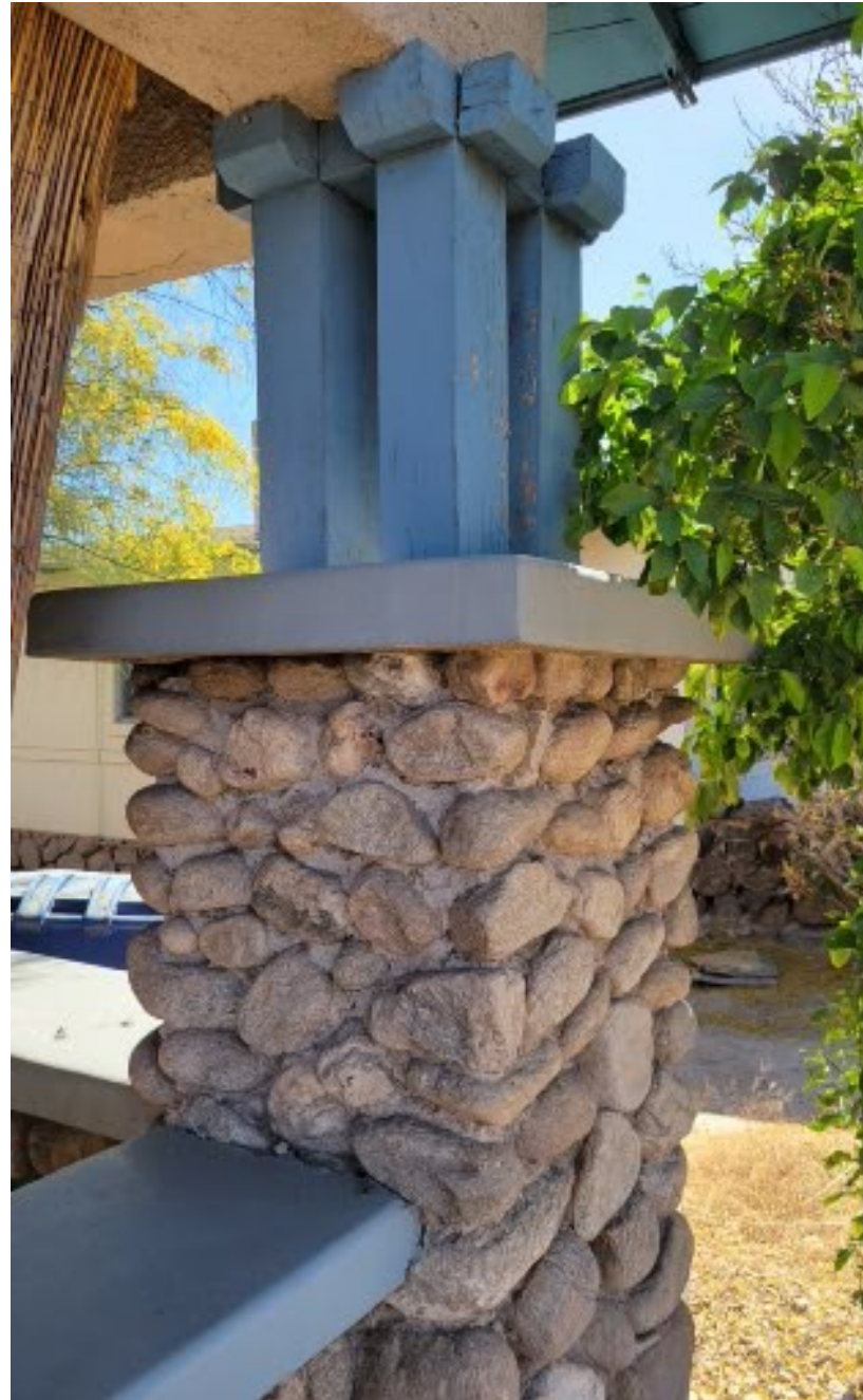
West porch pier, cobblestone base and clustered wood posts. Piers are 4" x 4.5"
