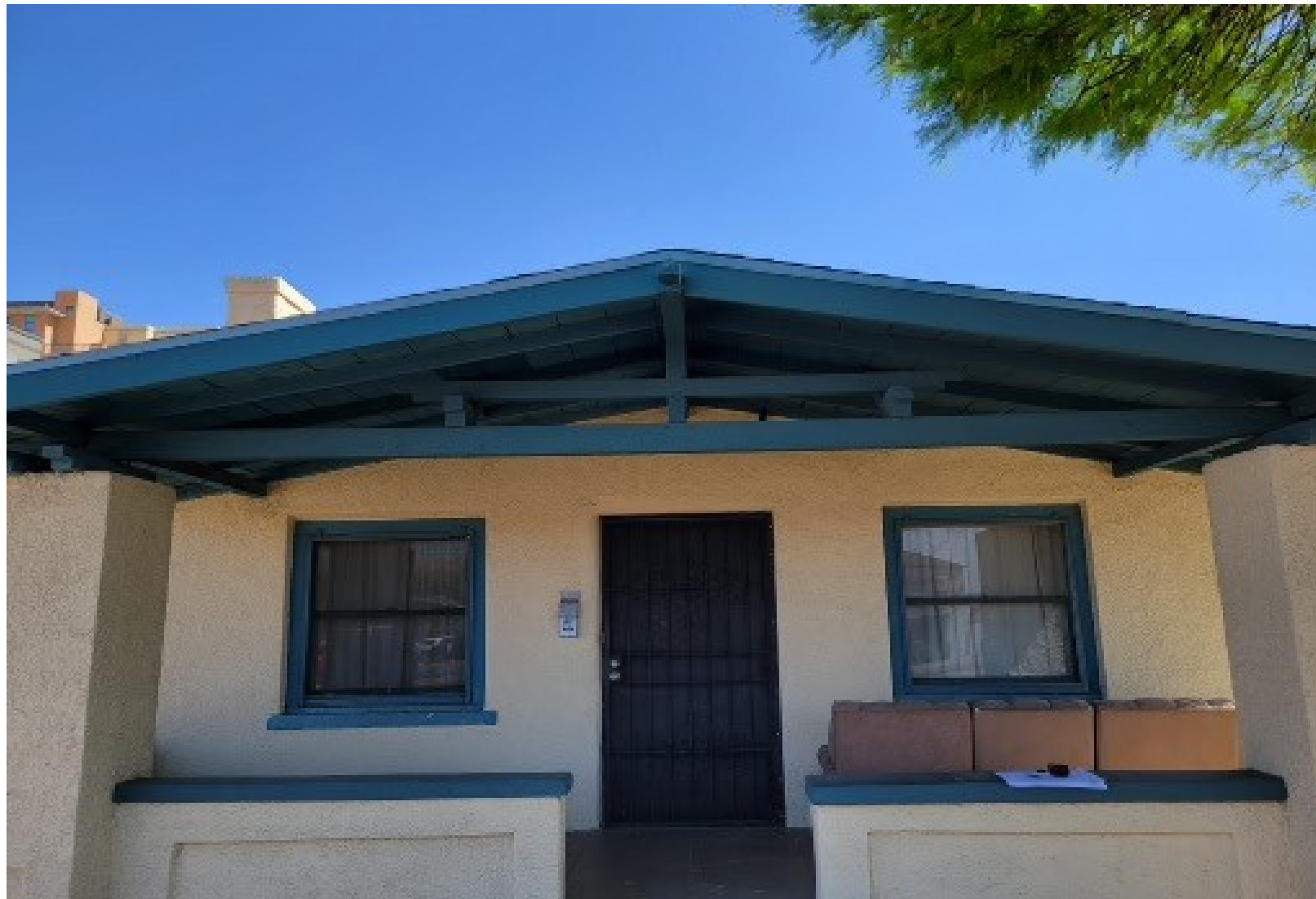
Looking at open truss in gable end, made of 4" x 4 "posts. The bottom chord is 4 x 6"
