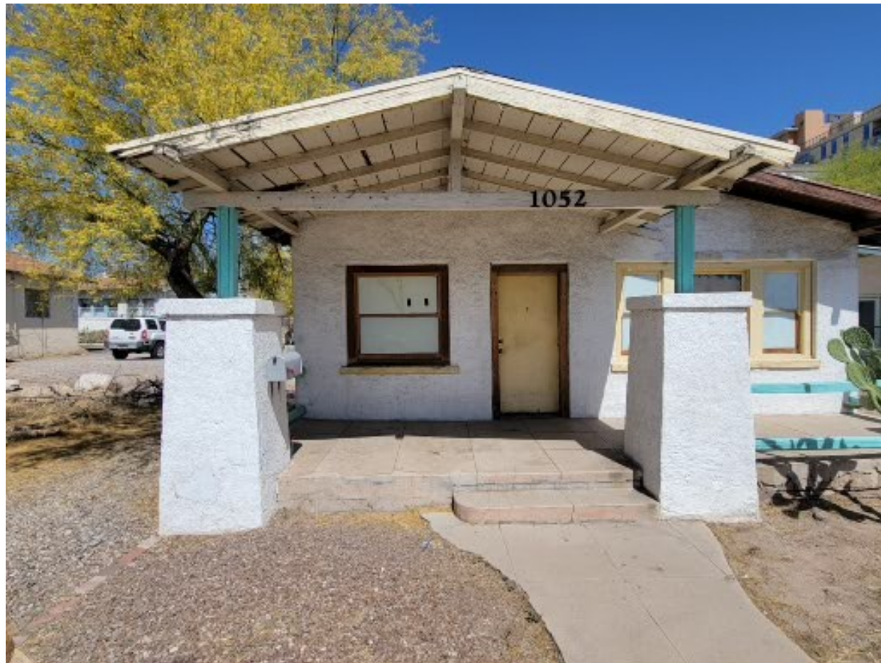
West facade. Very simple Craftsman piers and kingpost truss in porch gable.
