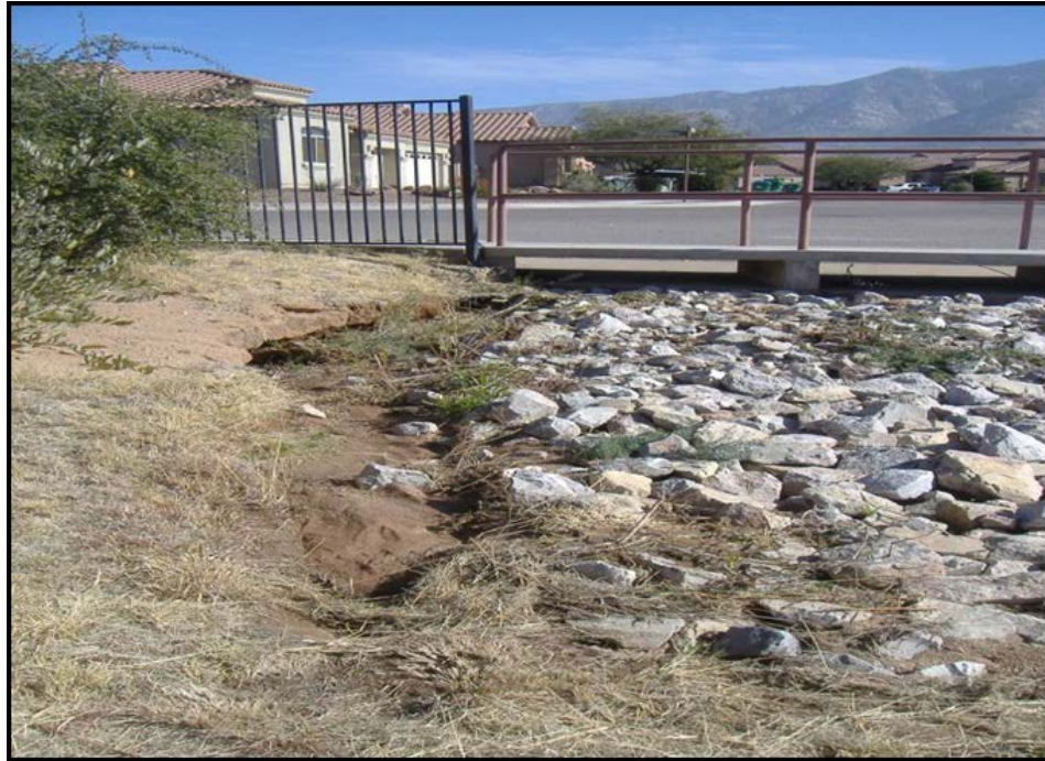
Photo 4.2 Basin Inlet with Inadequate Riprap Placement
