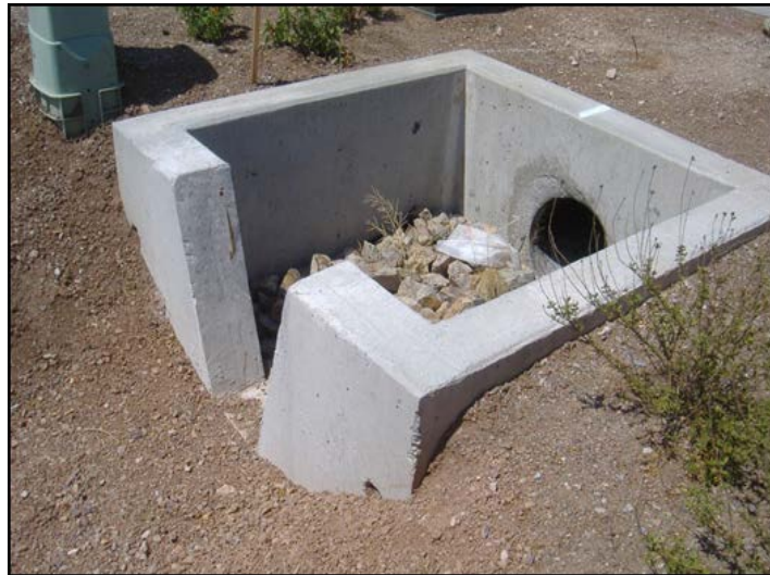
Photo 4.3 Combination Weir Box
