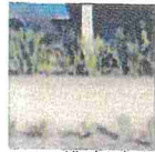
oxidized steel gate
