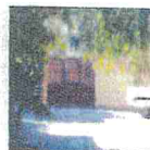
oxidized steel gate
