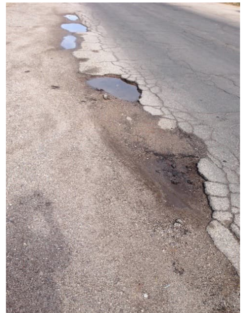
Figure 33: Increased pavement damage without curb.
