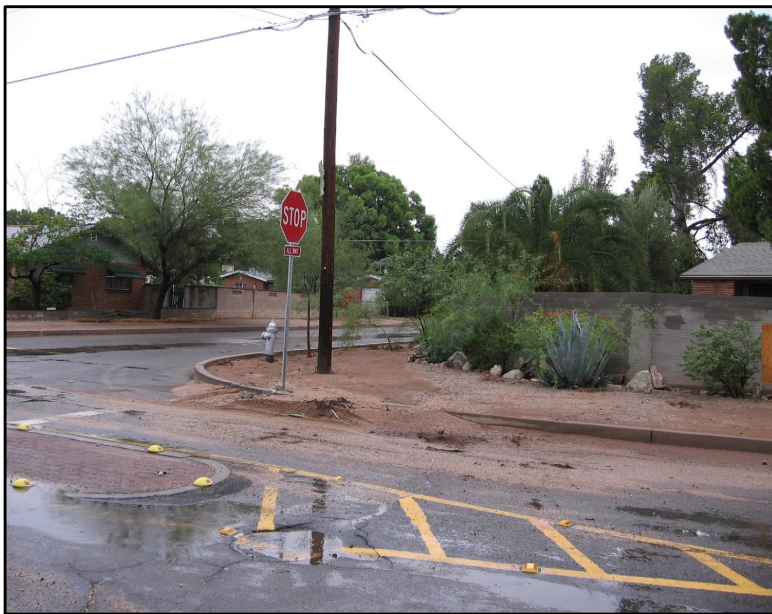
Figure 32: Erosion in right-of-way.
