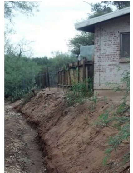
Figure 56: Erosion Hazards can cause structural issues
