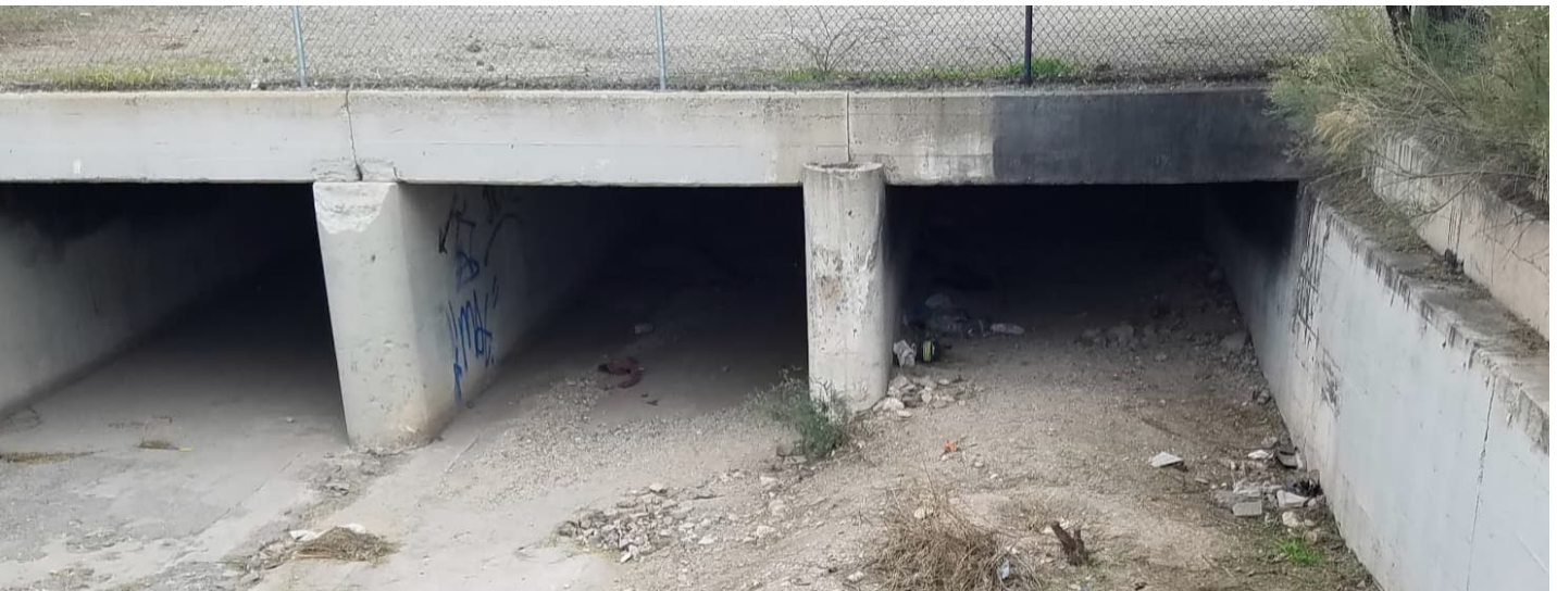
Figure 51: Blackened concrete at location where encampment was removed from box culvert after a fire.
