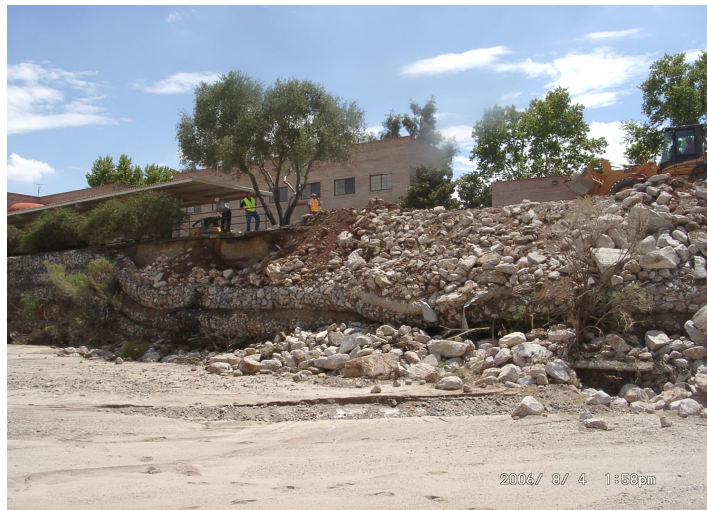
Figure 63: Flooding can easily damage city infrastructure
