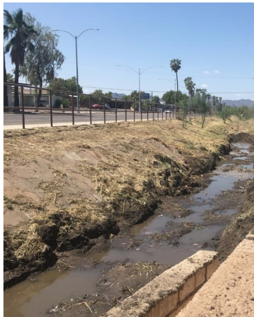
Figure 48: Maintenance is needed to re-establish flowline.
