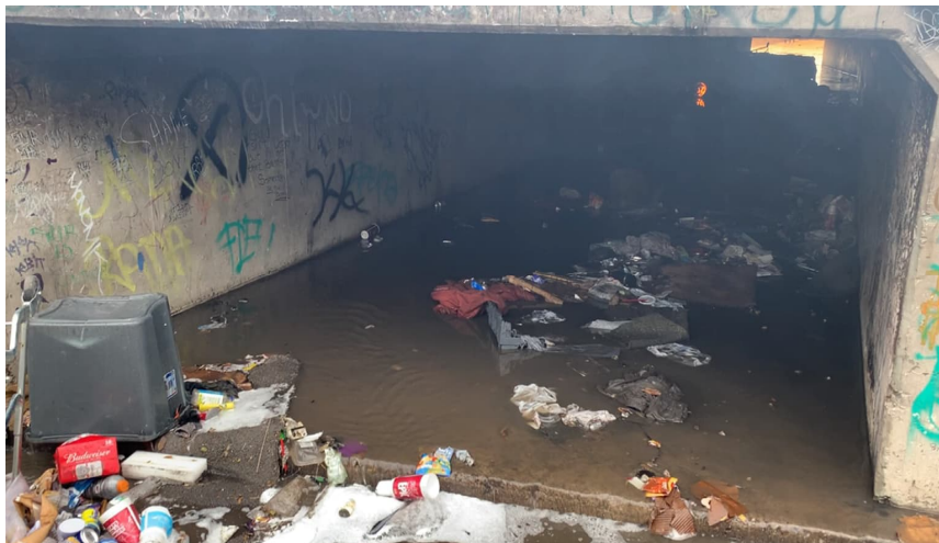
Figure 53: Fires in stormdrains cause potential pollutants and damage to infrastructure
